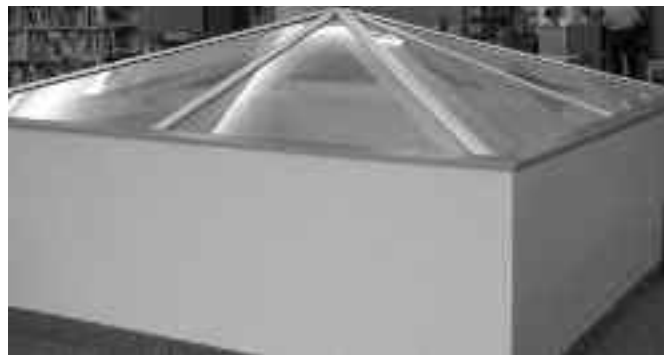
This skylight adds a dramatic touch to the new study area located on the second floor near the north side of the building.
